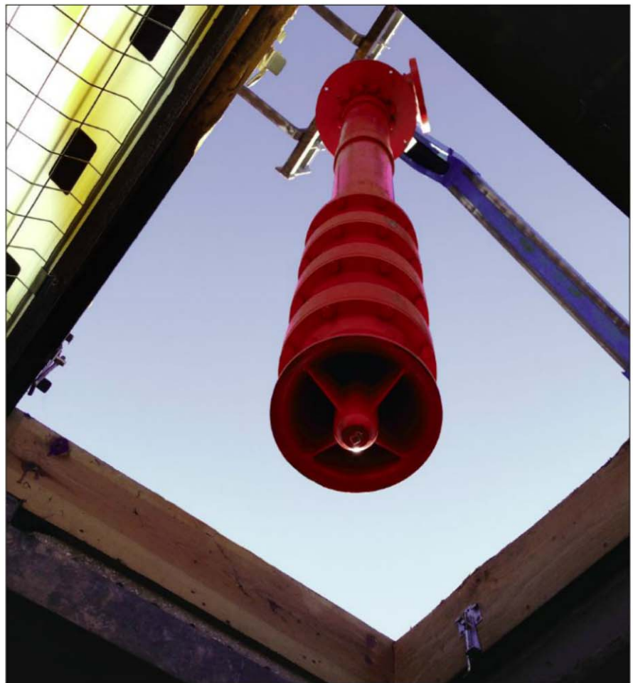
Jackson Associates hoisted the 20-foot-long shaft of a vertical turbine fire pump through the roof opening of a small building that is perched above an on-site, underground water reservoir.
