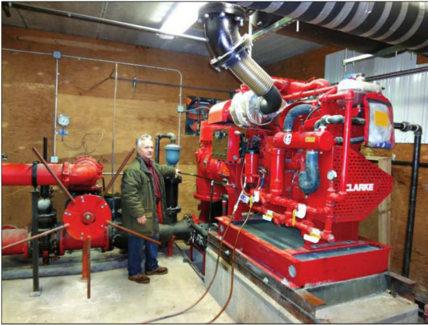
Jackson Associates President Rick Jackson surveys the new 530-horsepower diesel engine that serves as a companion to the vertical turbine fire pump.
